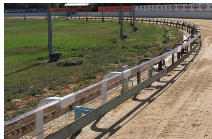
Traditional steel post & lure rail system with plastic safety rail used in SA
